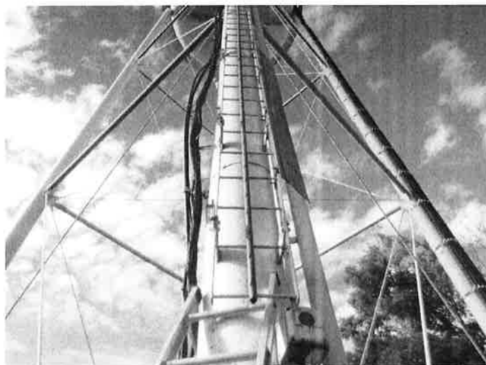
24) There is no vandal guard on the leg ladder.
