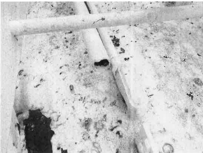
39) There are a few coating failures on the roof.
