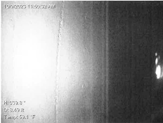
61) The wet interior sidewall coating is in fair condition overall.
