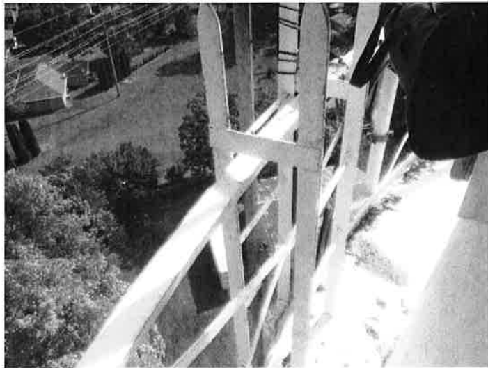
29) There is no opening in the balcony railing at the top of the leg ladder.
