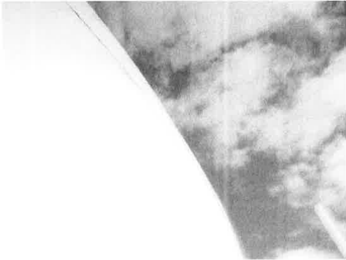
34) The sidewall coating is in good condition overall with a few areas of minor erosion.
