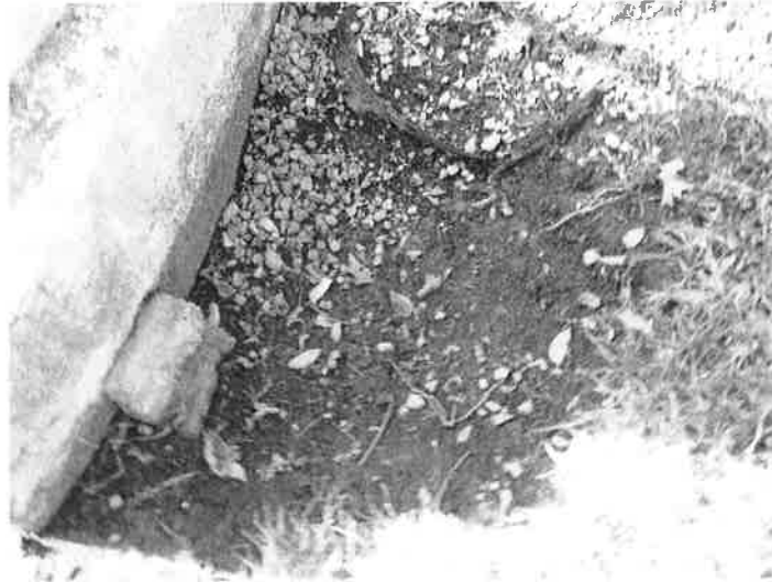
20) There is soil erosion around the leg foundation at the overflow pipe discharge.
