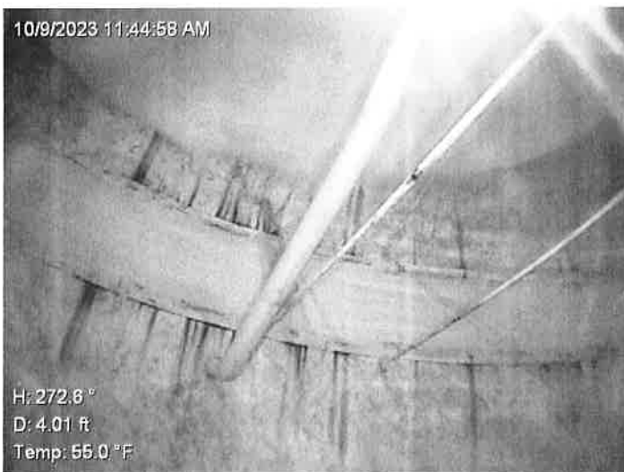
57) There are a few coating failures on the wet interior sidewall.
