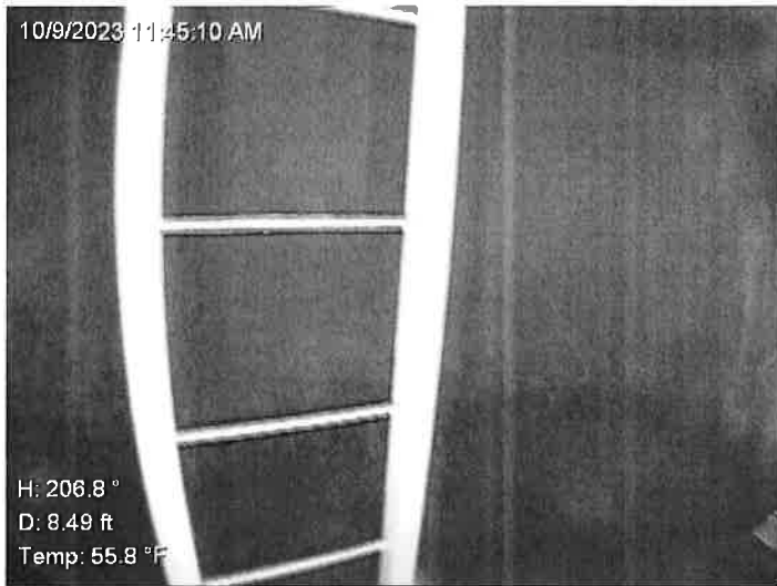
64) The wet interior ladder appears to be in good condition. The ladder is not equipped with a fall prevention device.
