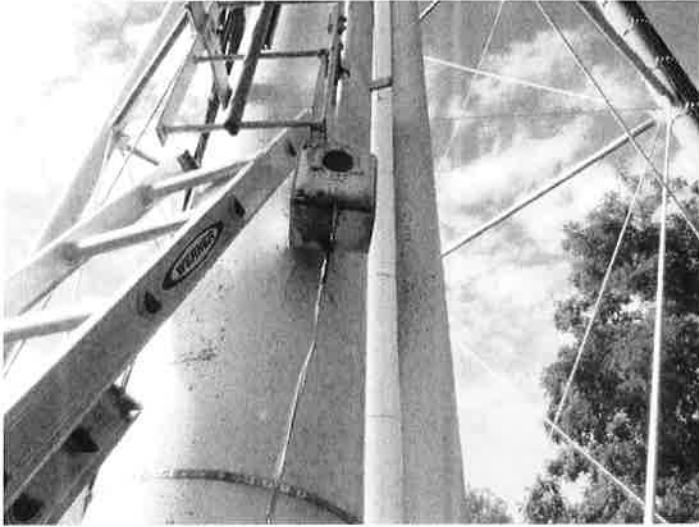
22) The photoelectric cell for the aviation light is mounted on a leg.
