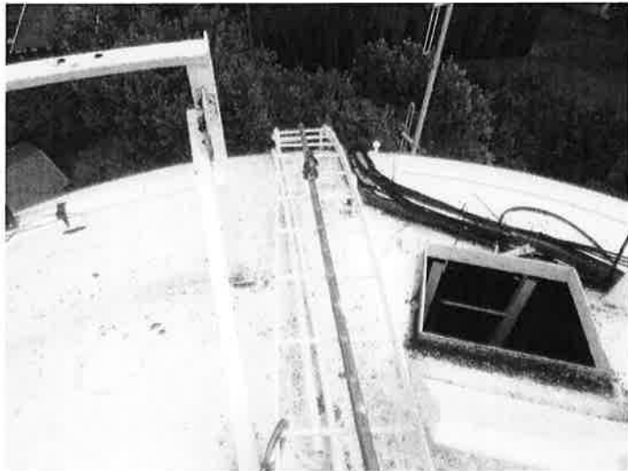
38) The sidewall/roof ladder is in good condition. The ladder is equipped with a fall prevention device.
