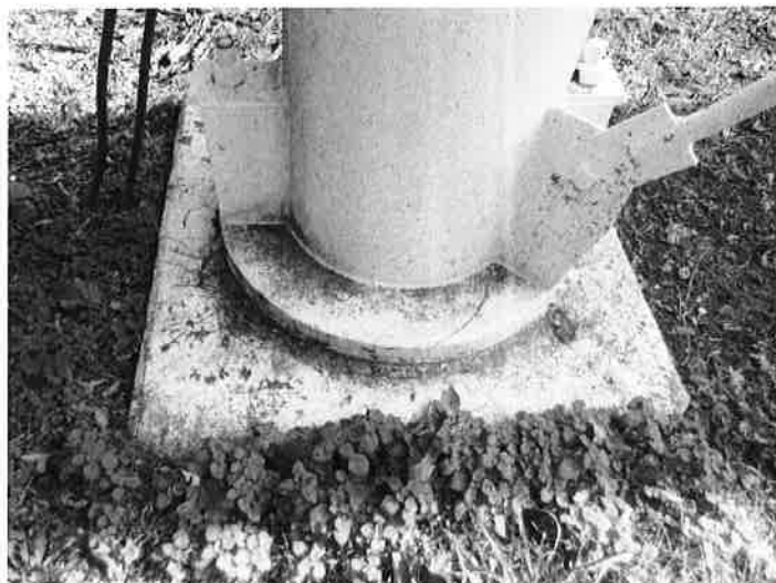
9) The concrete leg foundations are in good condition with no significant deterioration.
