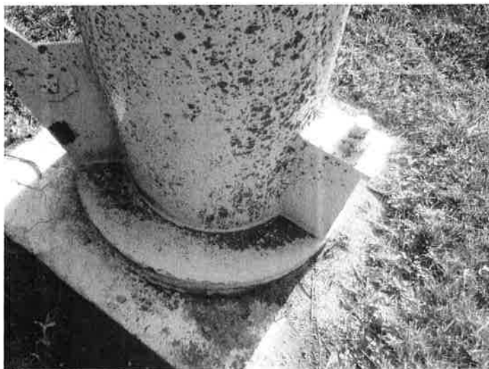
12) There are a few coating failures on the legs.
