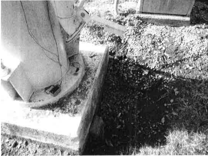
19) The overflow pipe discharges to the ground.
