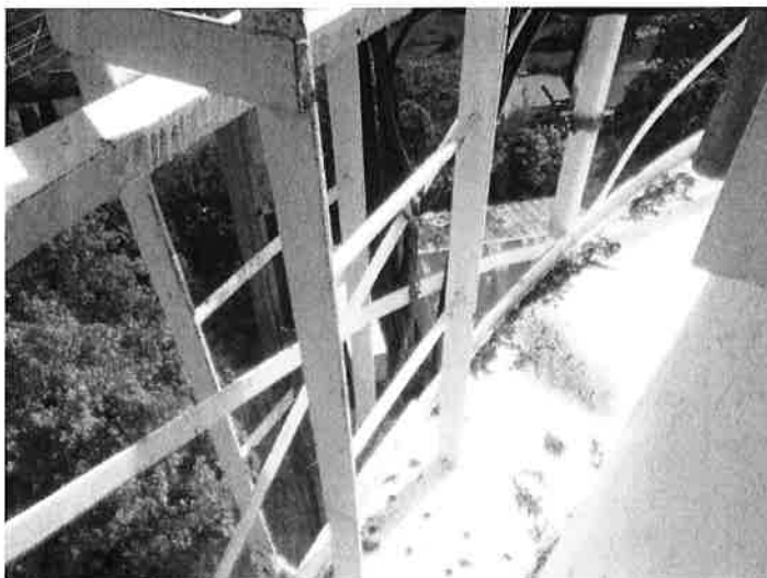
30) There is evidence of water ponding on the balcony.
