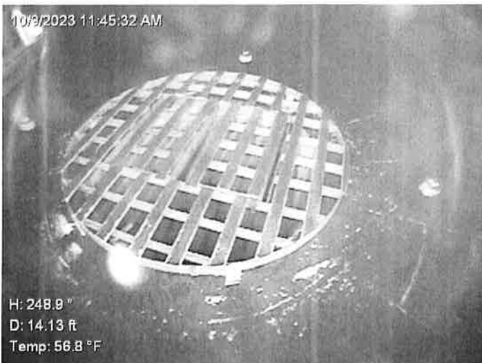
66) The grate over the riser in the wet interior is in good condition.
