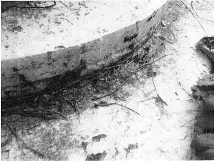
10) The grout between the steel leg baseplates and concrete foundations is intact.
